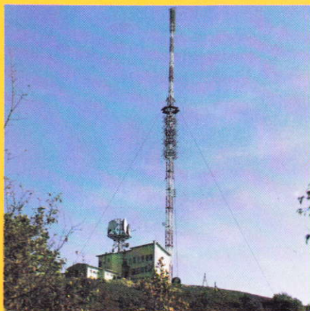
TV and VHF transmitter station with radio relay receiving antenna. Radio relay is often used as the feeder route in cases where cables would be difficult to lay.
